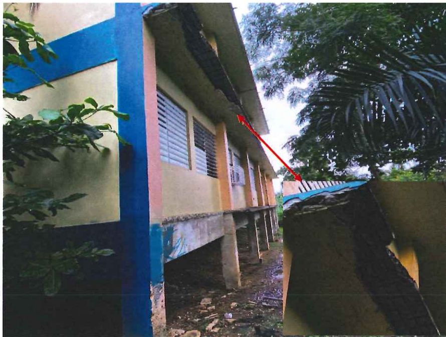
Photo 4: Exposed eave reinforcing bars
