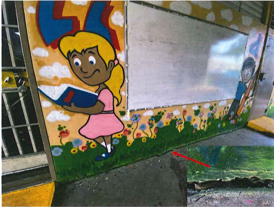
Photo 5: Crack on floor/wall intersection
