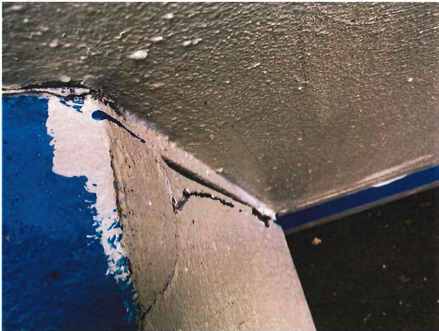
Photo 2: Crack at the side of the bridge
