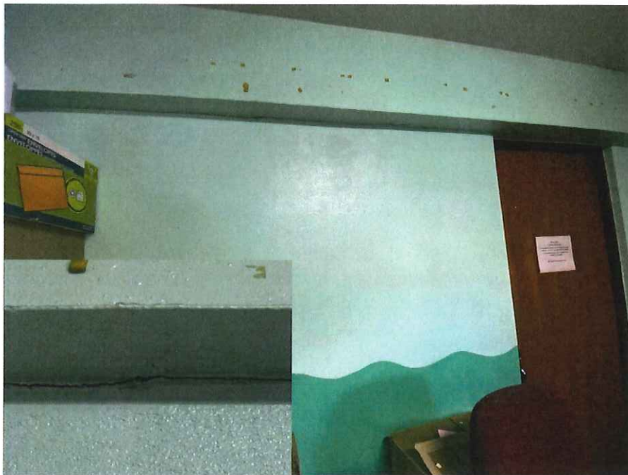
Photo 9: Crack wall/beam intersection
