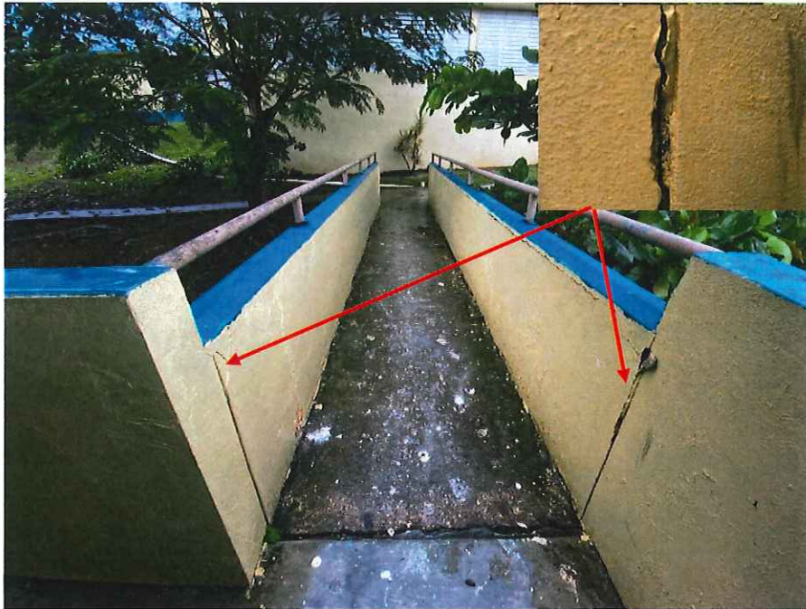
Photo 1: Crack at both sides of the bridge
