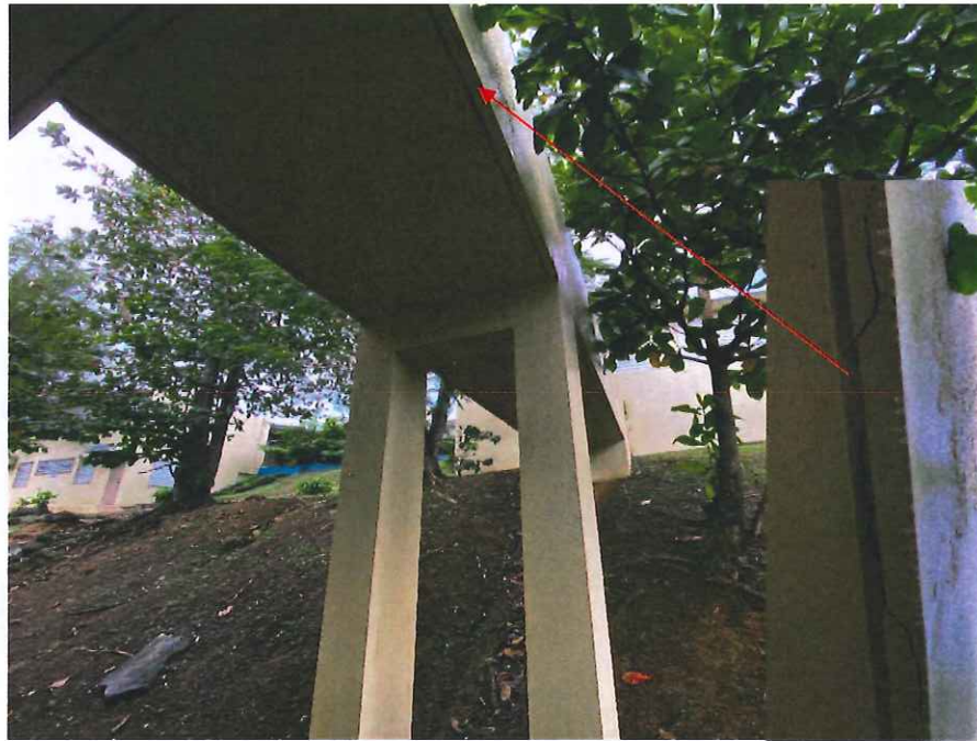
Photo 3: Crack under the bridge
